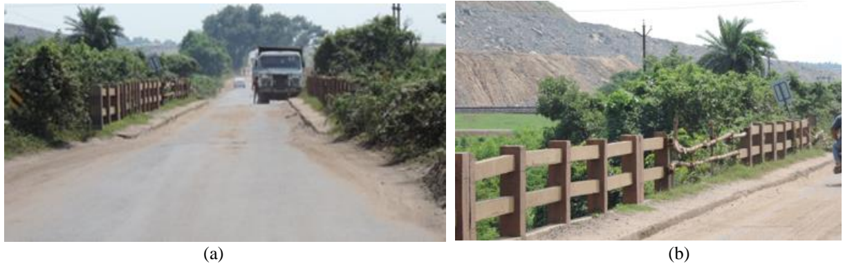
Fig. 6. Safety Issues at Narrow Bridges (a) No proper signages and dense vegetation (b) Broken parapet wall
