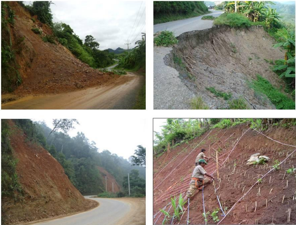
Figure (10). Landslip and remedial works in Laos
