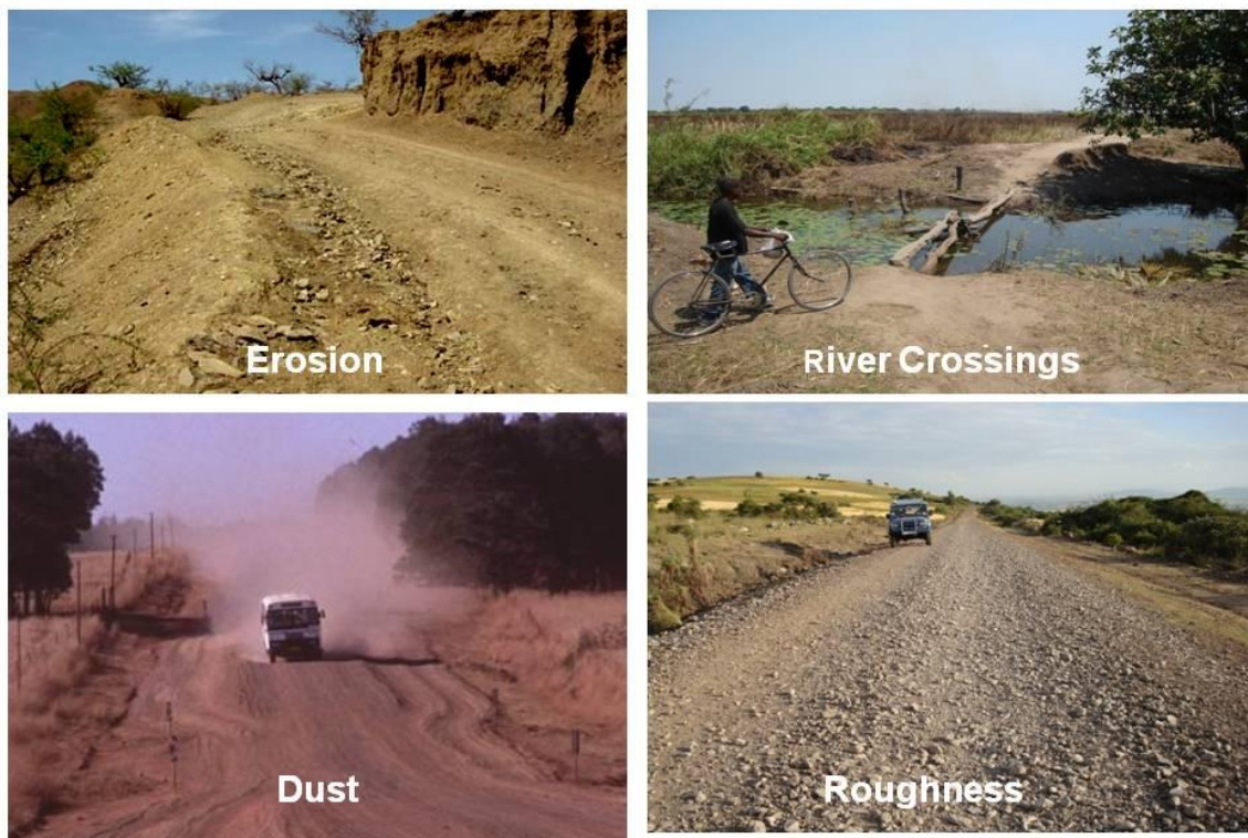
Figure1. Typical problems on gravel road networks
